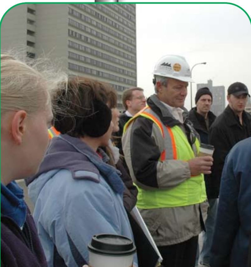
Peter Sanderson, Project Manager for Flatiron•Manson, leads interested community participants on a tour of the construction site from the 10th Avenue Bridge.
